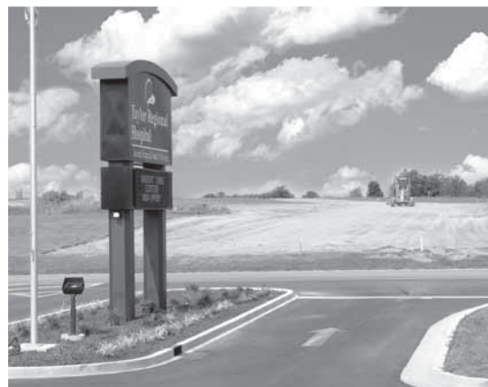
Construction is nearing completion on the road leading to the future Taylor Regional Medical Park Complex.
